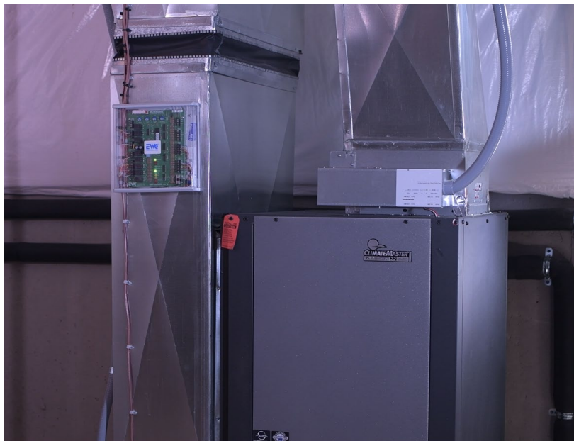
ClimateMaster Tranquility Heat Pump System Installed April 2023
