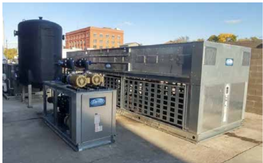
Recent installation of a Drake brewery chiller system.
